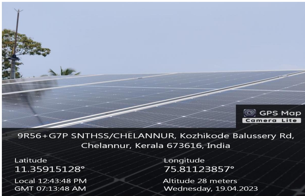
Figure 19 SOLAR POWER PLANT IN THE COLLEGE
